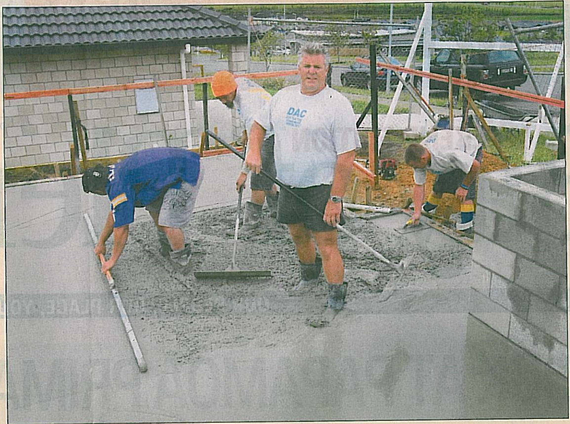
GROUNDWORK: Concrete contractor, Dean Anderson, lends a hand at the Waipuna Hospice fundraising house at the Lakes subdivision. PICTURE / JOHN BORREN 031209JB07BOP
