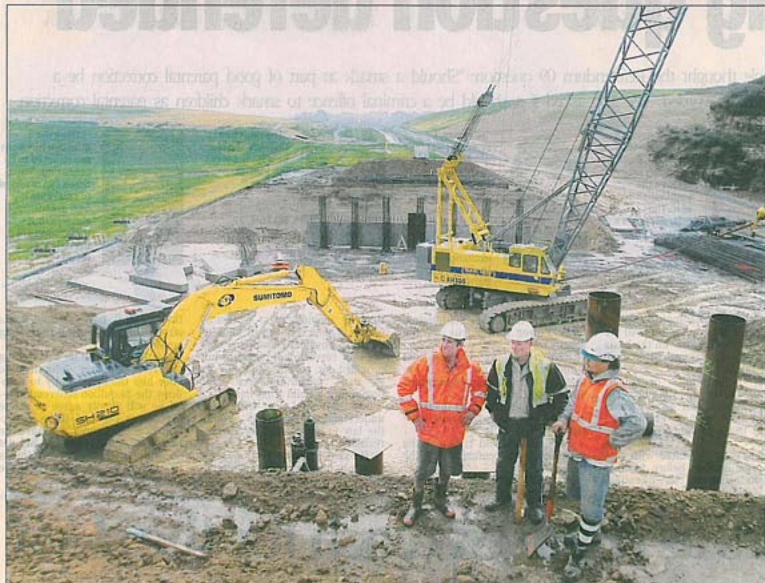
SPAN UNDERWAY: Spartan Construction's Peter Littleton, Grant Hume and Sam Hurna at the site of the new bridge being built by the developer of The Lakes to provide access to the subdivision. PICTURE / JOHN BORREN 120609JB068OP
